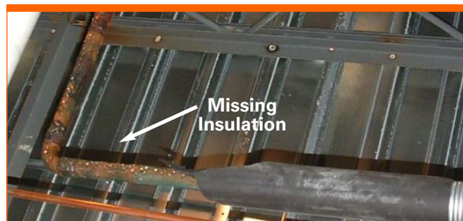
Figure 10 – Missing Suction Line Insulation
