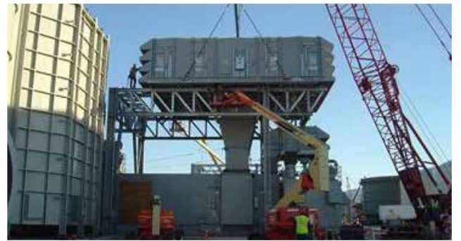
The clearcurrent systems work with all turbine types. Examples of installed projects include a GE 7FA turbine (above), as well as an GE LMS100 aeroderivative solution (above).
