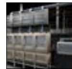
Valve Manifold Boxes (VMBs)
