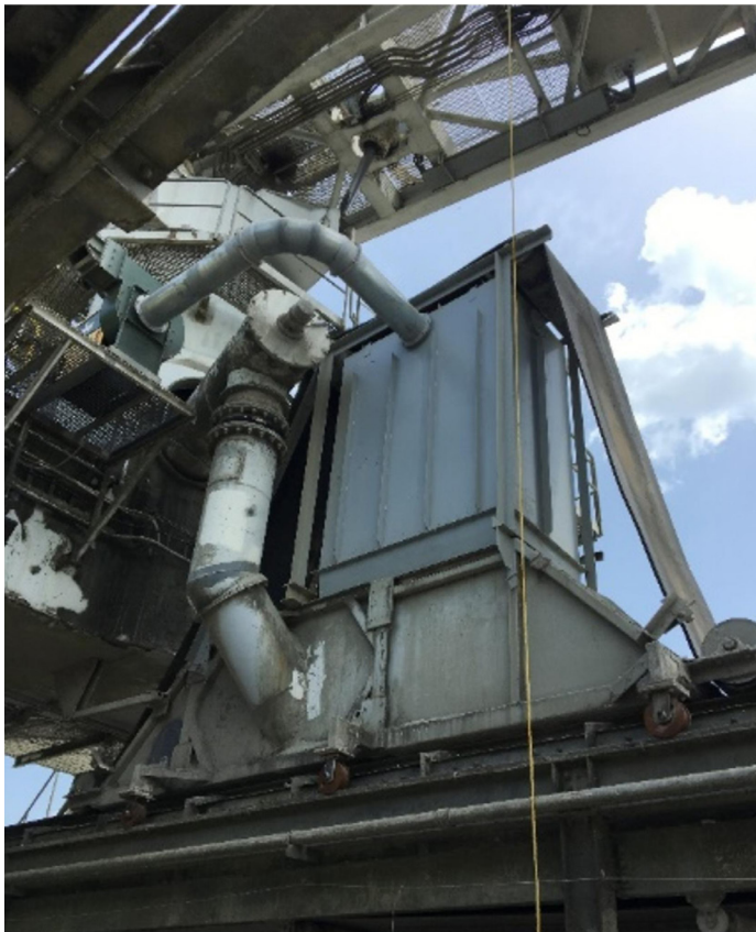
Figure 5. Customised new dust collector on top of BC-1 loading chute.
