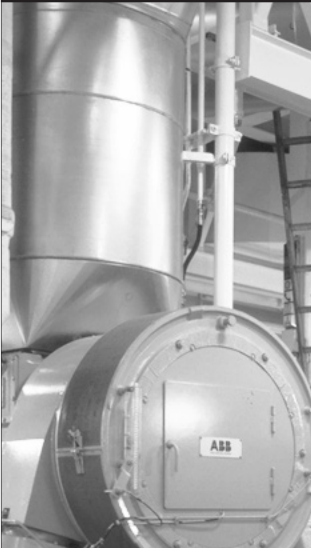
FUEL & LUBE OIL CABINET
