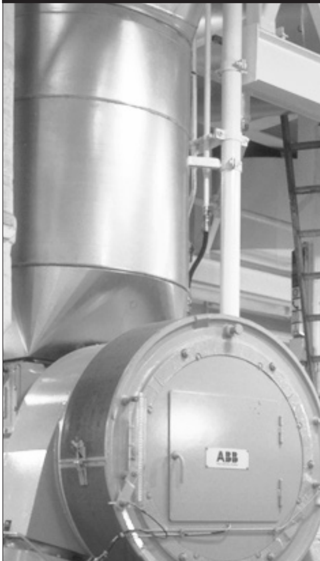
FUEL & LUBE OIL CABINET
