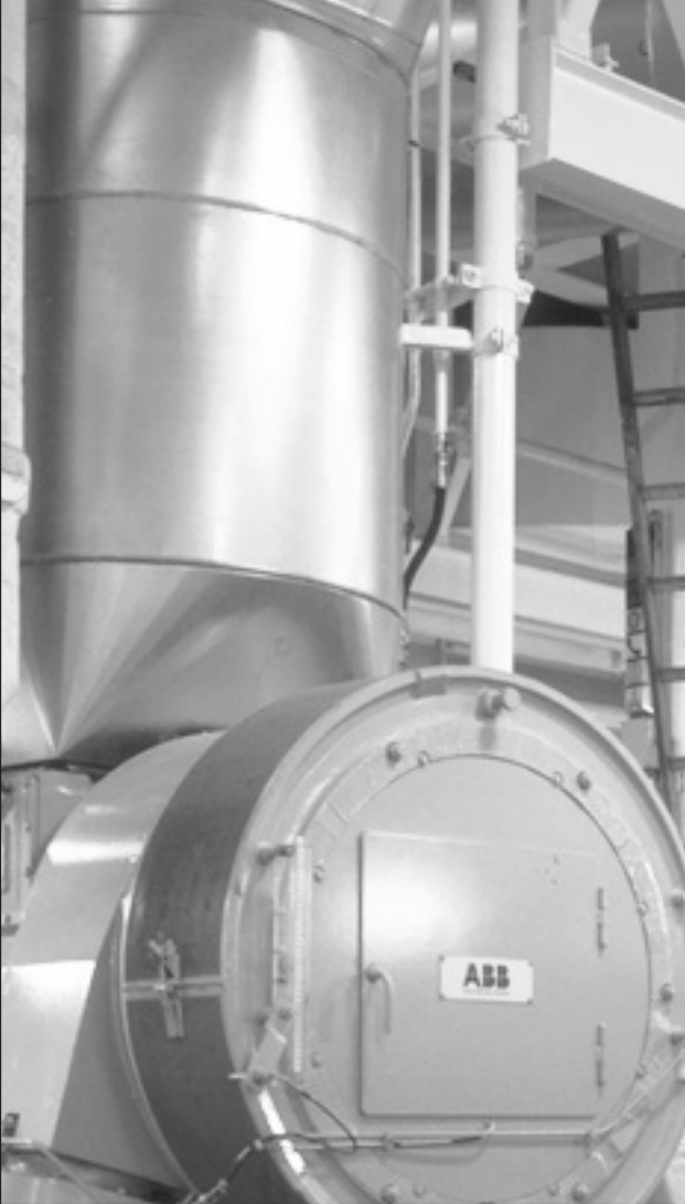
FUEL & LUBE OIL CABINET
