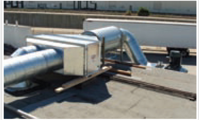
Exhaust duct from the DustHog SFC downward flow dust collector with in-line silencer and safety filter.
