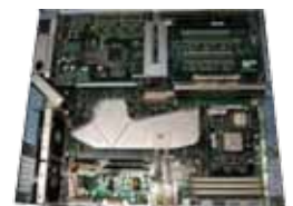
Switch and routers
